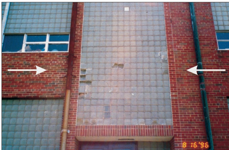
Figure 29 The long, continuous brickwork intersects the vertical glass block wall. Pressures have broken the glass blocks in line with the long continuous expanse of brick work.
